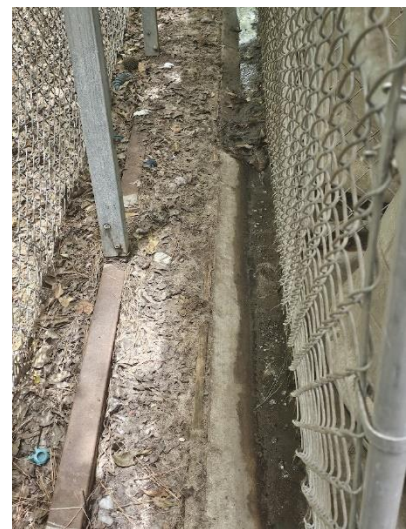
Back kennel drain clogged due to lack of preventative maintenance
